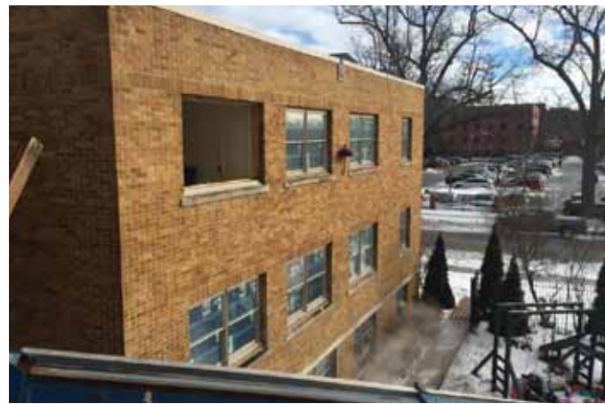
New window installation is nearly complete. A total of 99 new windows were installed. This adds additional comfort, efficiency and safety to the Women's, Children's, and Family Shelter.
