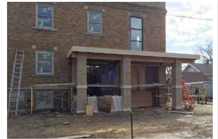
Masonry work is nearing completion. The new entrance will be handicap accessible and will offer greater security as guests enter the shelter. The entrance will be covered to offer relief from the elements, and will be monitored by security cameras.
