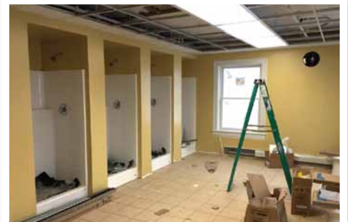
Fresh primer and paint is starting to go on to the walls to give everything a fresh new look. We can't wait to show you the finished project! Stay tuned!
