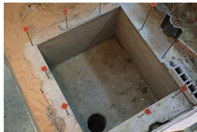
The beginning stages of the new elevator shaft being constructed. The elevator has been relocated to be more useful and accessible to our guests and staff.
