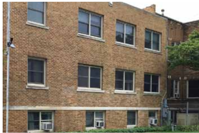
The windows in the building were decades old and in need of replacing. They allowed heat to escape and cold air to enter into the building and rooms.
