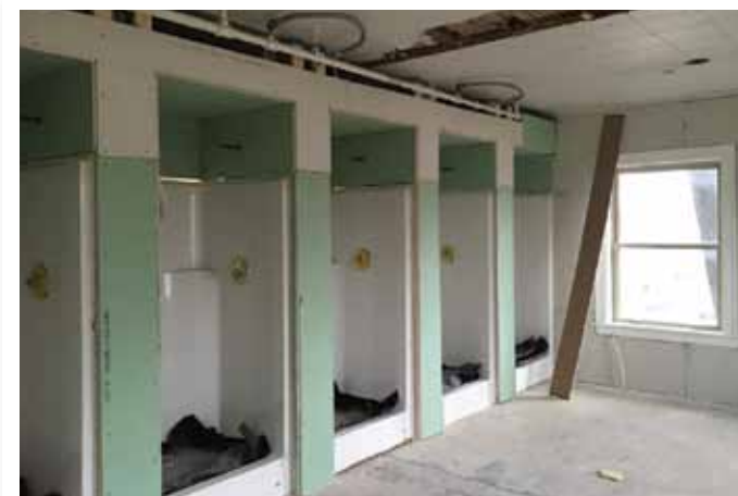
The bathroom facilities have been expanded. This photo shows the shower stalls cased in with drywall. The updated restroom facilities will be a great addition to the shelter.
